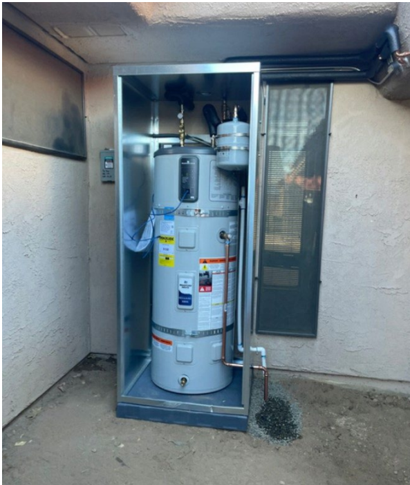
Figure 33. Heat Pump Water Heater Installed at the Bartz–Altadonna Community Health Center
