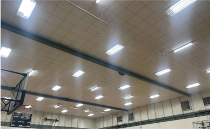
Figure 4. VUSD – De Anza High School Gym LED Light Replacements
