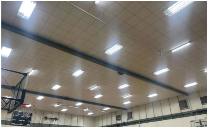
Figure 28. VUSD—De Anza High School Gym LED Light Replacement
