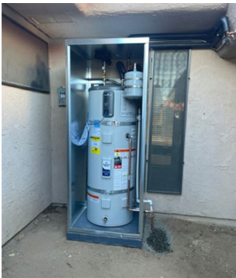
Figure 5. Heat Pump Water Heater Installed at the Bartz–Altadonna Community Health Center
