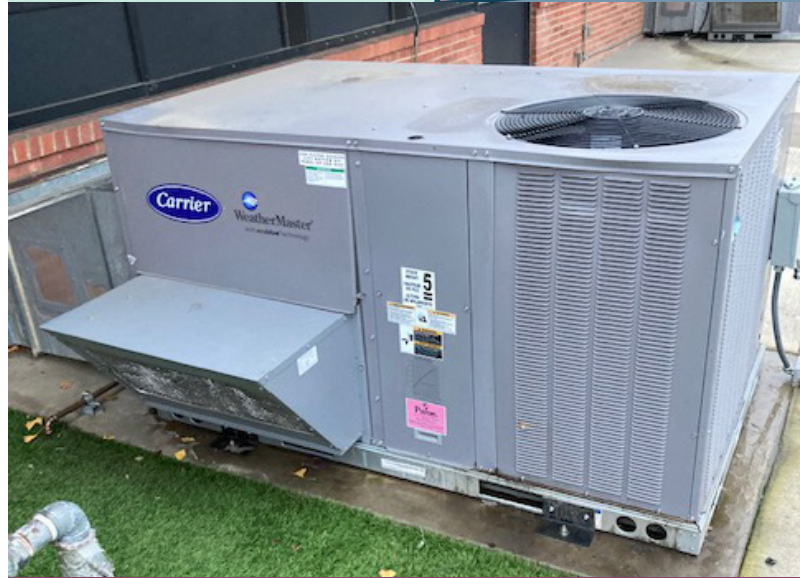
Heat Pump HVAC system installed at West Putnam Elementary school library.
