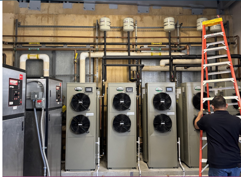
Picture: Heat pump water heaters installed in UCI Health medical facilities, Orange, CA.
