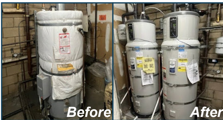
Before and after photos of one of the water heater replacements at City Yard.
